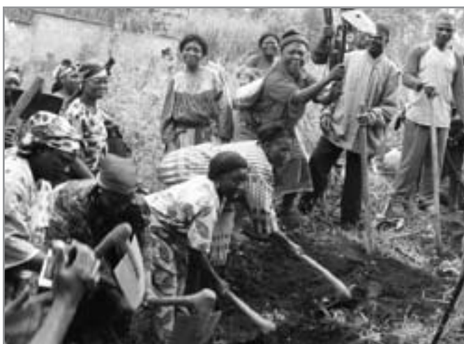
Workers from 11 villages in Wum, Cameroon pitch in to help work on the water project that is sponsored, in part, by Grace Church, Keswick.
